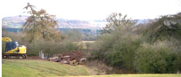
Larches on the embankment of the Shropshire Union canal, with Peckforton Hills in background (and repairs in the foreground!)
